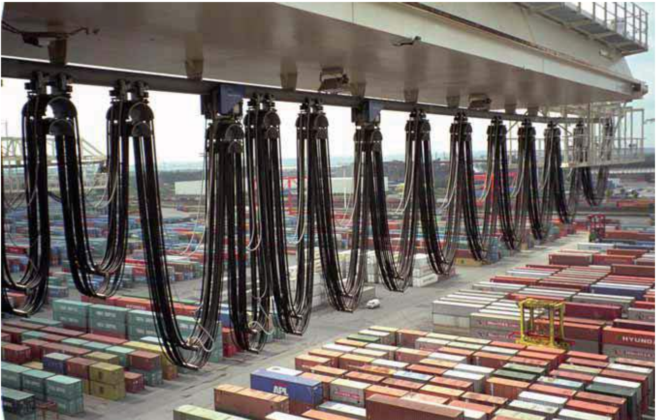
Motor driven VAHLE Cable Carriers, Hamburg Harbour
